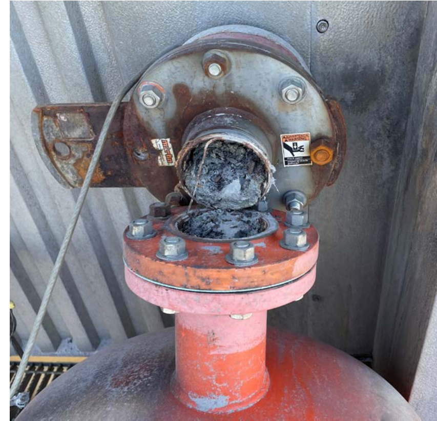
Corrosion from Positive Pressure System
