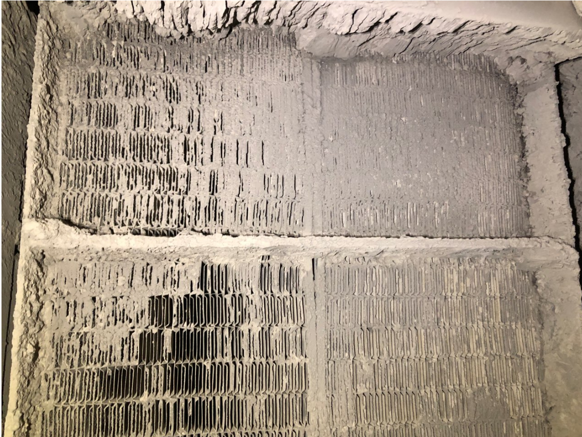
LPA Underside of Unit 5 SCR – Steam Event
